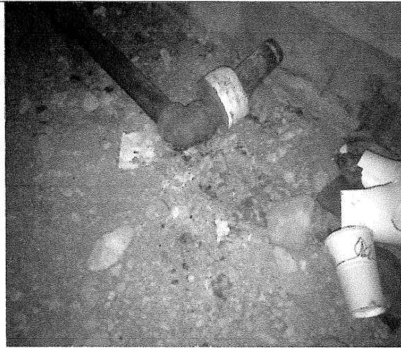
Photo #7: TSI debris on floor in tunnel
