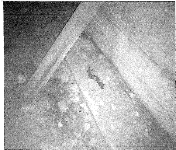
Photo #8: TSI debris on floor in tunnel
