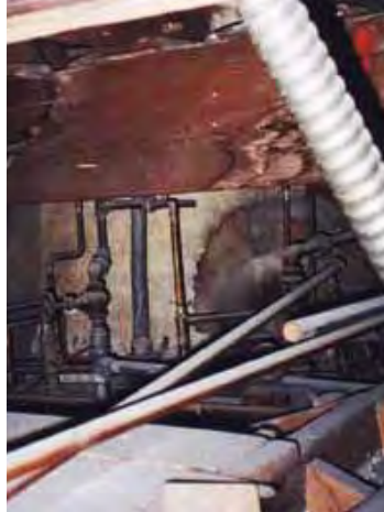
Aging infrastructure between floors
