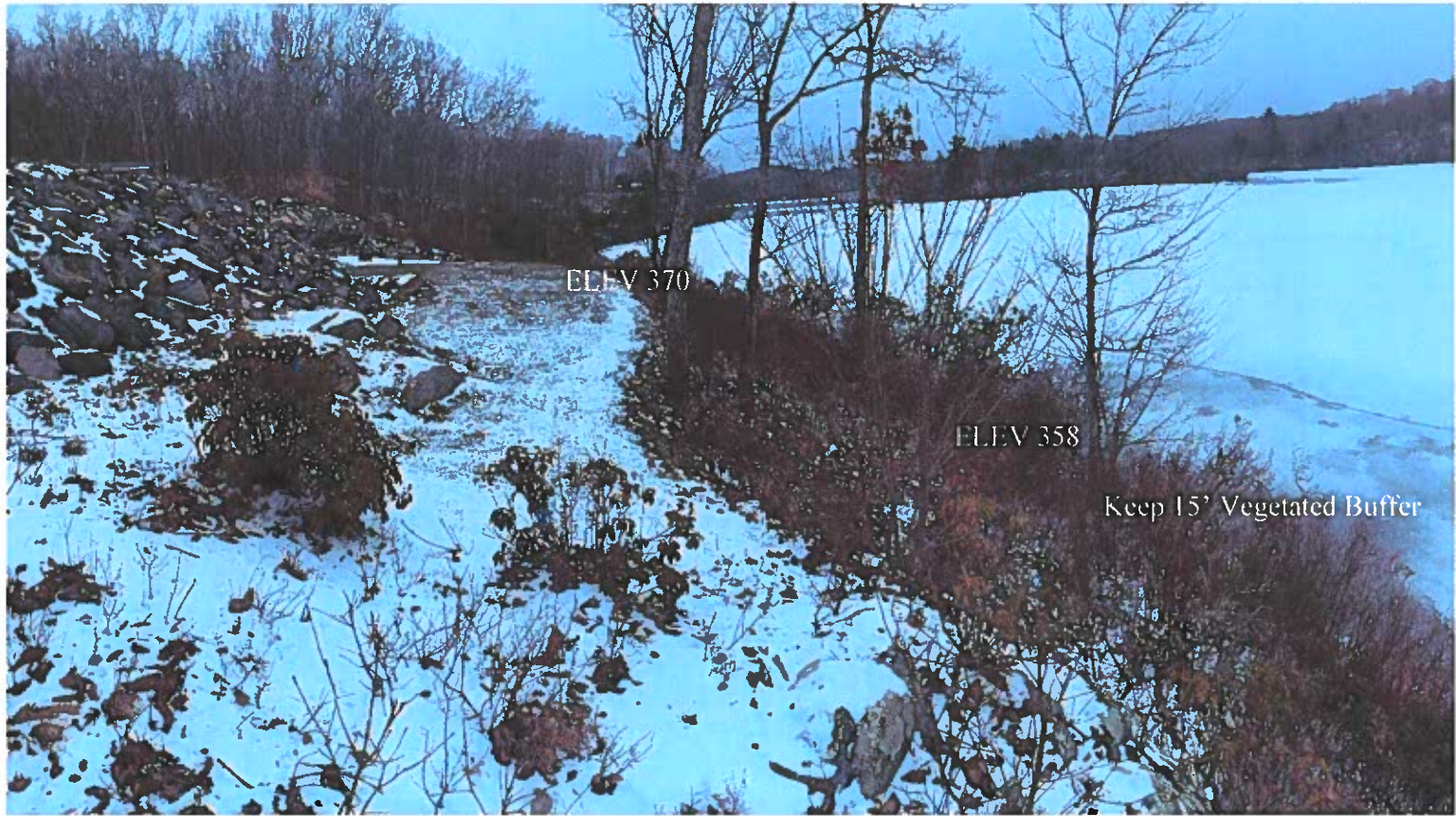
Photo 2: Top of existing terrace which is proposed to be excavated to match lower-level grade or expose ledge.
